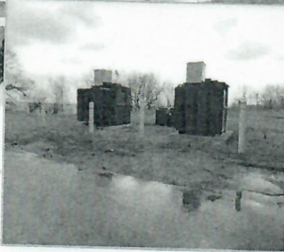
TYPICAL PAD MOUNTED TRANSFORMER
